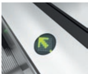
LED traffic lights located in the decking
